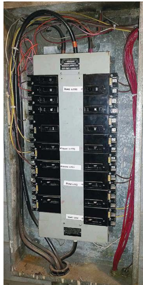
Photo 2. No equipment grounding conductors (EGCs) originate from the lighting distribution panel (shown here) to the lighting control panel (not shown).
