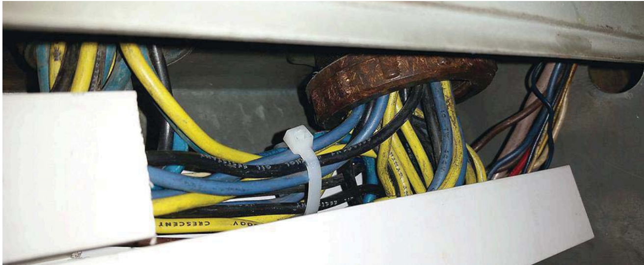
Photo 1. No equipment grounding conductors (EGCs) were pulled from the lighting branch circuit pull box to the individual AC lighting branch circuits.
